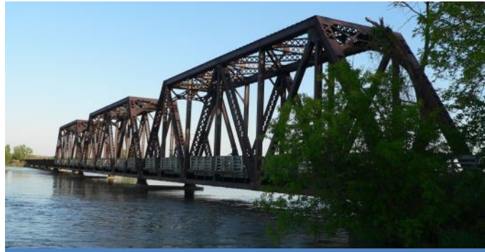
Photograph 6.3 Niobrara River Bridge (Destroyed in March 2019 flooding) Source: Nebraska Historical Society
