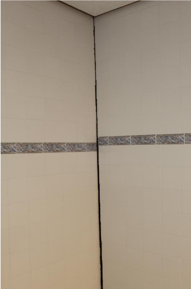
Photograph 13.4 Example of Subsidence and Plasticity in the Lake Area. Block basement wall.
