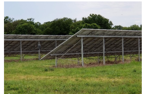
Example of a Solar Conversion System, Ground-mounted
